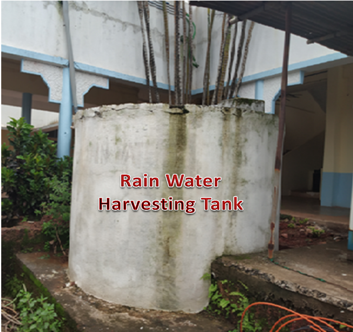
Rain Water Harvesting Tank
